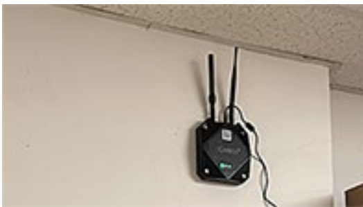
Figure 6. Gateway installed in the manager's office near the mechanical room.
