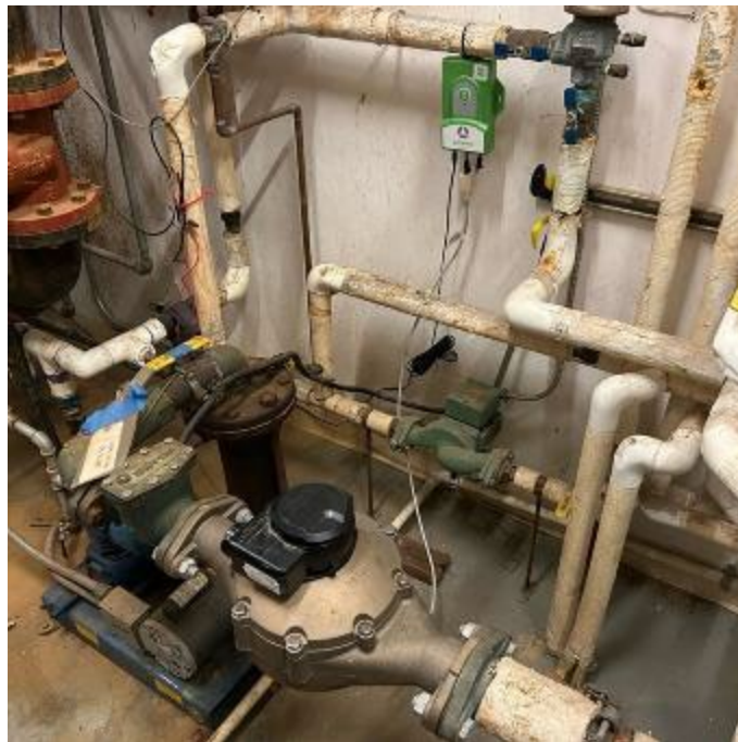
Figure 9. Domestic cold water (DCW) supply to the store with the Evolution Utility Meter Sensor attached.
