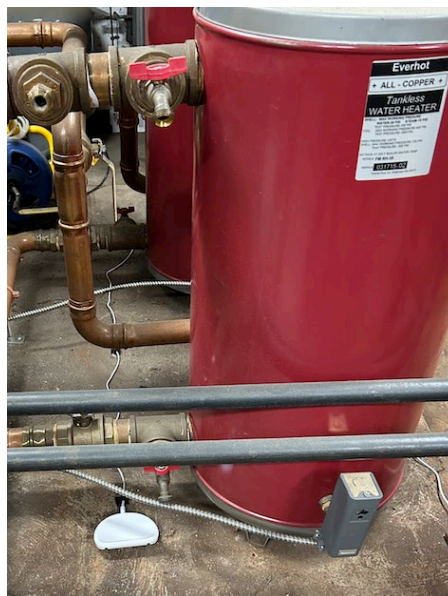
Figure 12. Evolution puck and rope leak sensors near water heater tanks.
